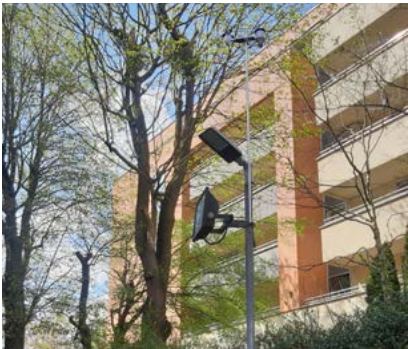
Weather station installed on a streetlamp at Liceum Akademickie Da Vinci at a height of about 3 meters above the ground
