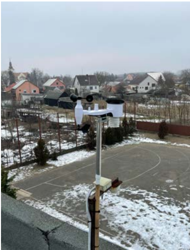
Weather station installed on the rooftop of Szent Piroska Greek Catholic Primary School, Hungary
